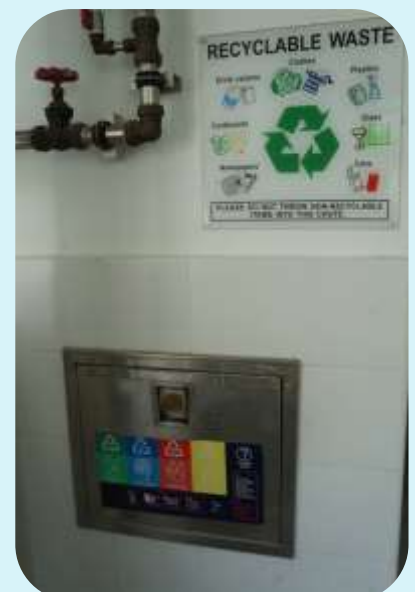
Recycling chute at Treelodge@Punggol
