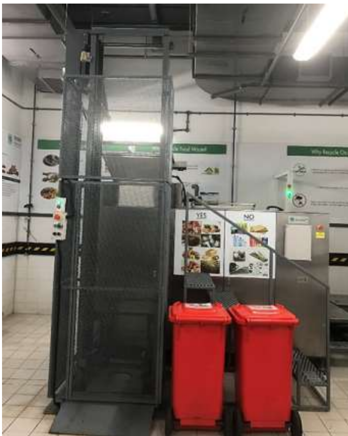
Food waste treatment system at Our Tampines Hub
