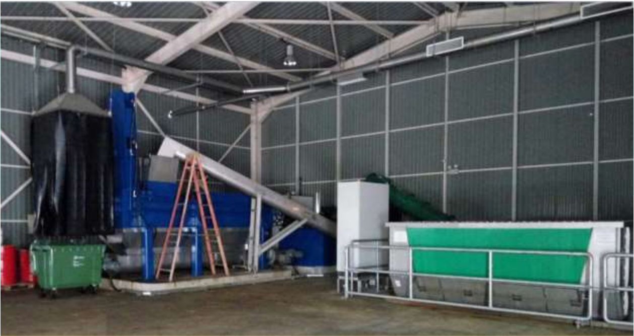
Pilot food waste and used water sludge co-digestion project
