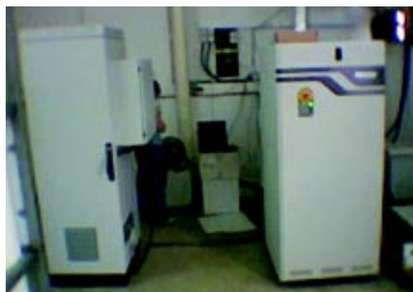
Fuel cell power system in Pasir Ris carpark
