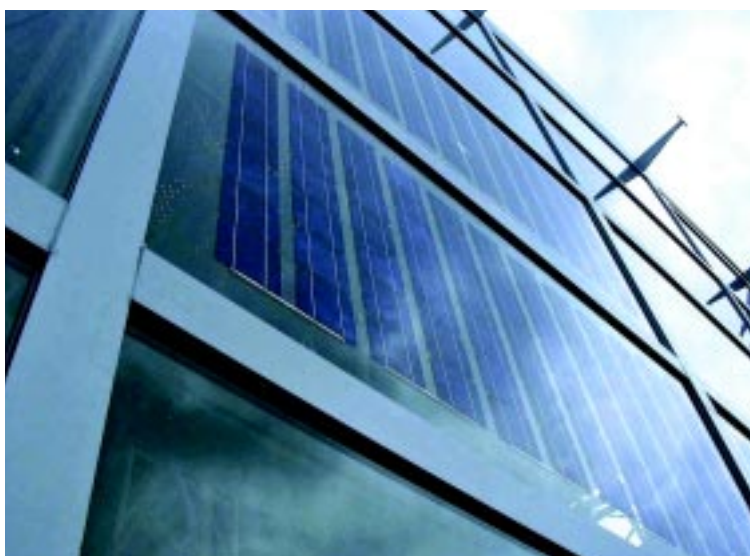
Building integrated photovoltaics at Biopolis Visitor Centre
