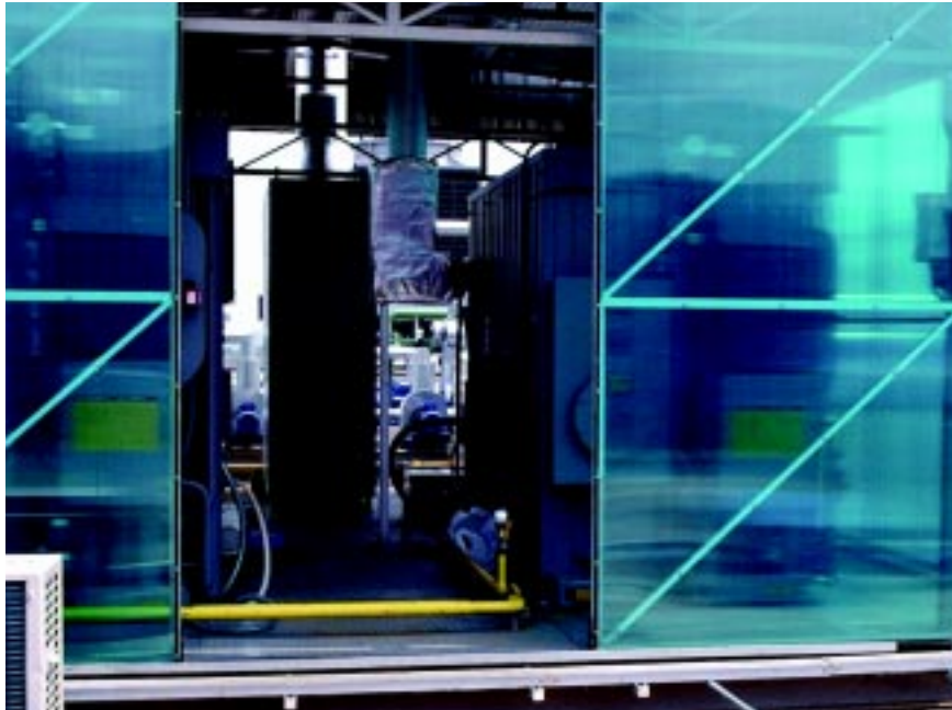
Trigeneration system at a food manufacturing plant in Tuas
