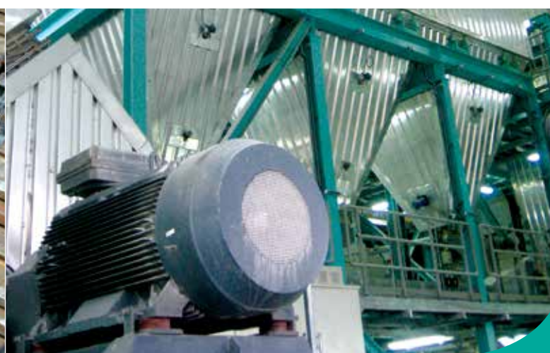
Flue Gas Treatment
