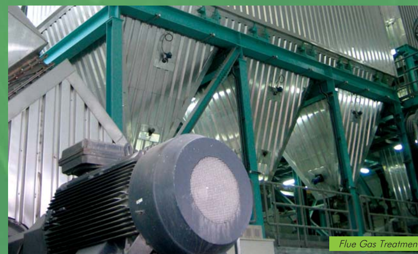
Flue Gas Treatment
