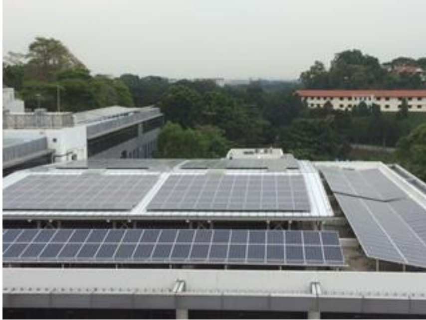
Figure 1: Solar PV panel on the roof top of high-rise buildings
