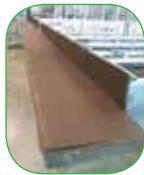
Protective layer of padding along the platforms off the conveyor systems
