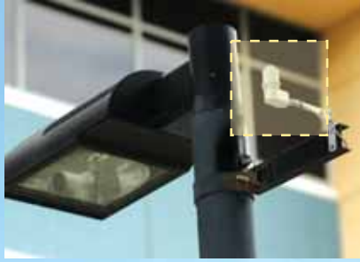
Rain sensors cut off irrigation during heavy rain
