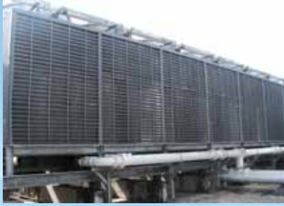
Cooling towers use NEWater
